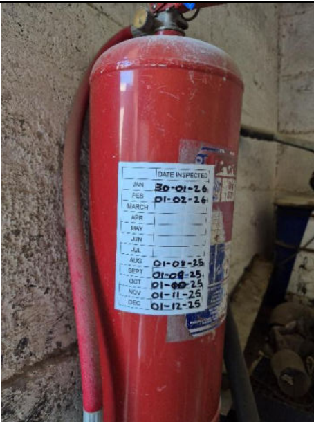
Fire extinguishers on site
